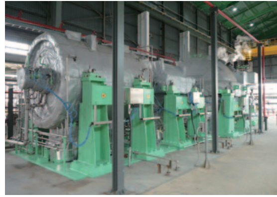
3 Charge gas compressor
