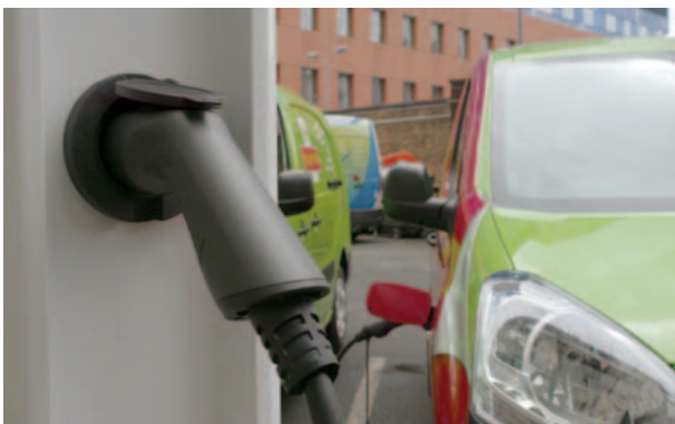
Figure 5 | EV Plugged into Charging System
