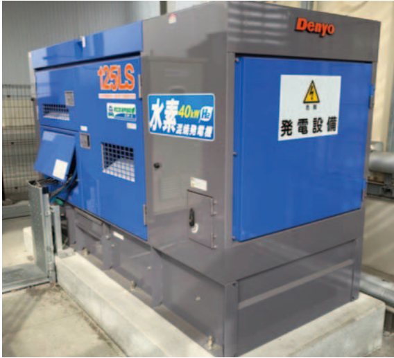
5 Hydrogen mixed fuel generator
