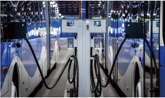
[13] Electric buses charging devices implemented at the Vasteras depot in Sweden
