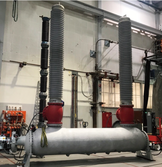
Breaker (GIS) during SLF90 Testing at Accredited STL Laboratory.
