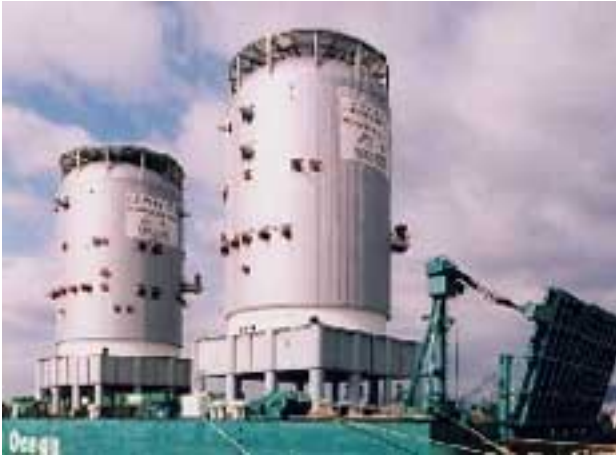
Fig. 2— Twin-Furnace Boiler (“W.B.”) of the Power Station.
