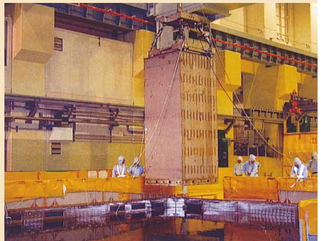
New high-density BSS rack installed in SFP
