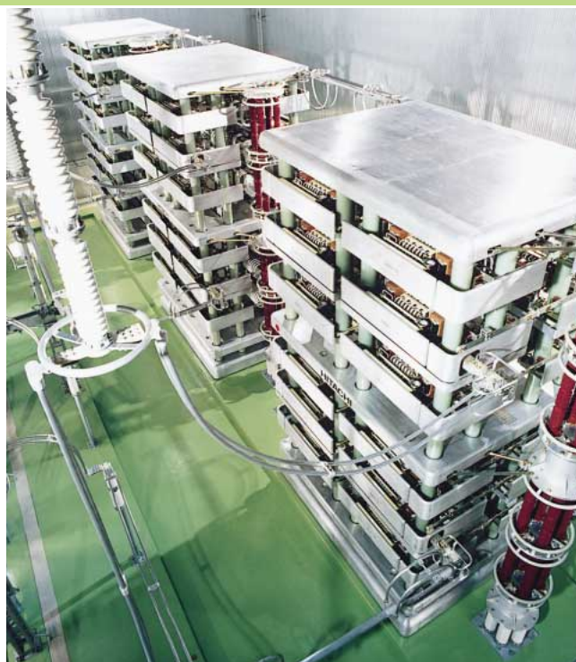
The 700-MW thyristor valve (250-kV/2,800-A quadruple-valve unit)
