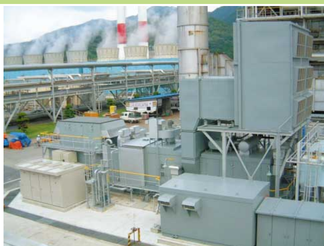
H-25 gas turbine at LGPC Yosu Plant
