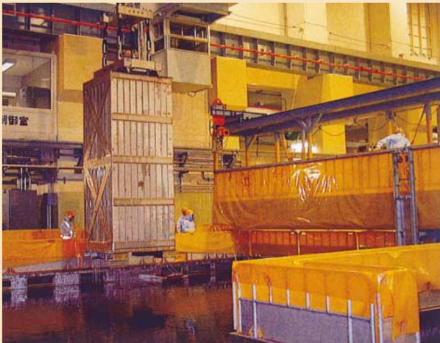
Existing stainless-steel rack detached from SFP
