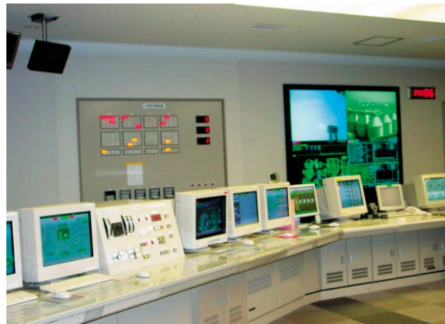
Fig. 4—Main Control Room of Shinko Kobe No.2 700-MW Power Station.
